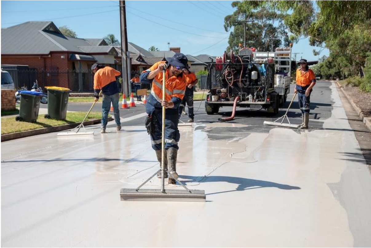
Some councils are experimenting with lighter-coloured road surfaces. (Supplied: City of Charles Sturt)
