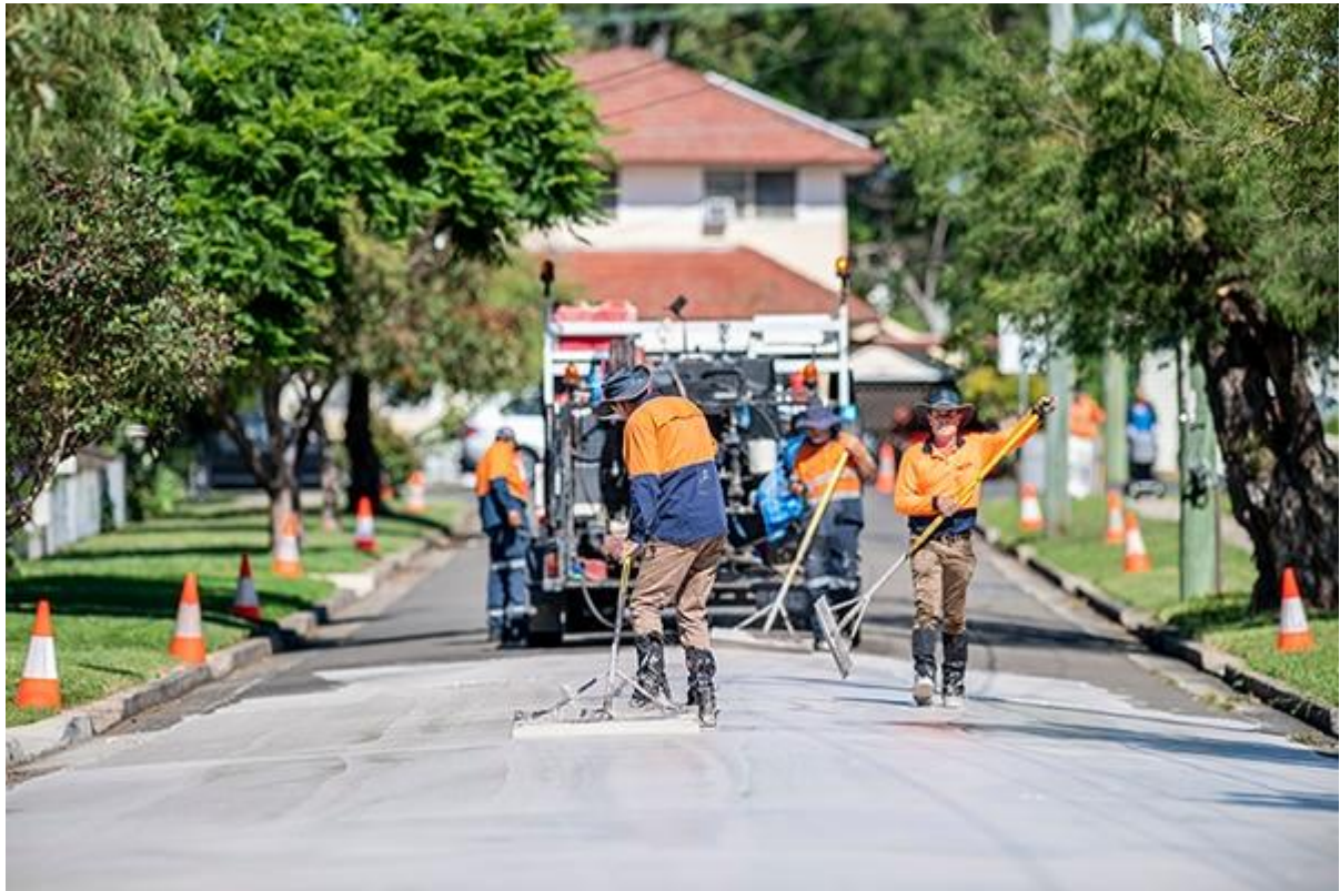
CoolSeal being installed in Western Sydney in March 2020. (Supplied: City of Paramatta/George Gittany Photography)
